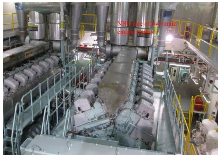
NBD one of two main engine rooms
